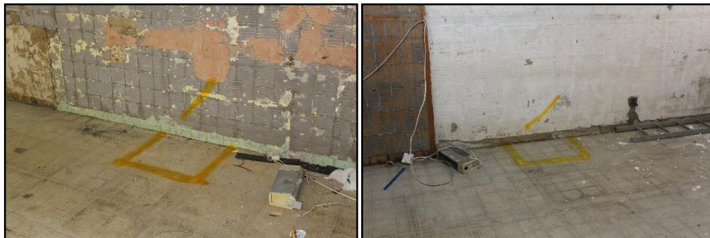
(Figs 7 & 8 – HSG21-WB Test Pit 1 Location on the left, Test Pit 2 Location on the right)
